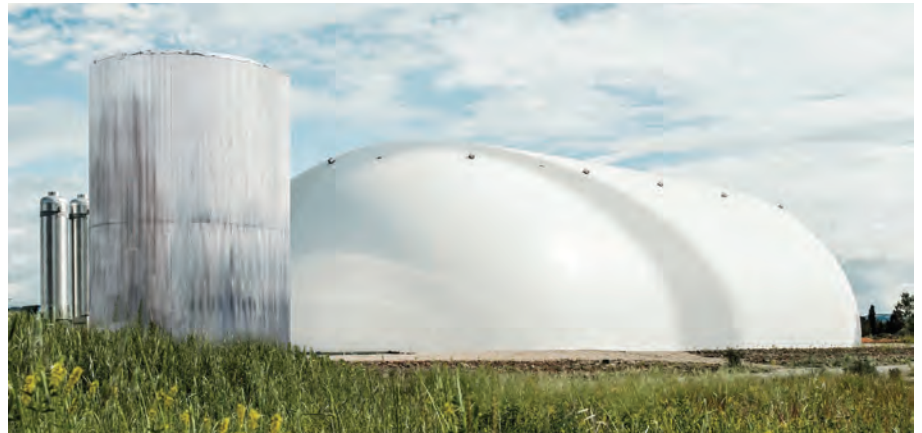
Energy Dome’s CO 2 battery located in Sardinia, Italy. Photo courtesy of Energy Dome.
